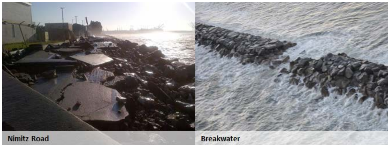
Figure 2: Port of Long Beach Damage from Hurricane Marie in 2014
